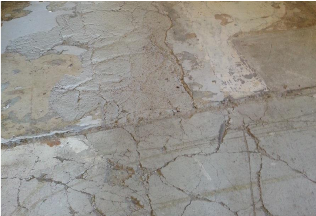
Distressed Gypsum subfloor
